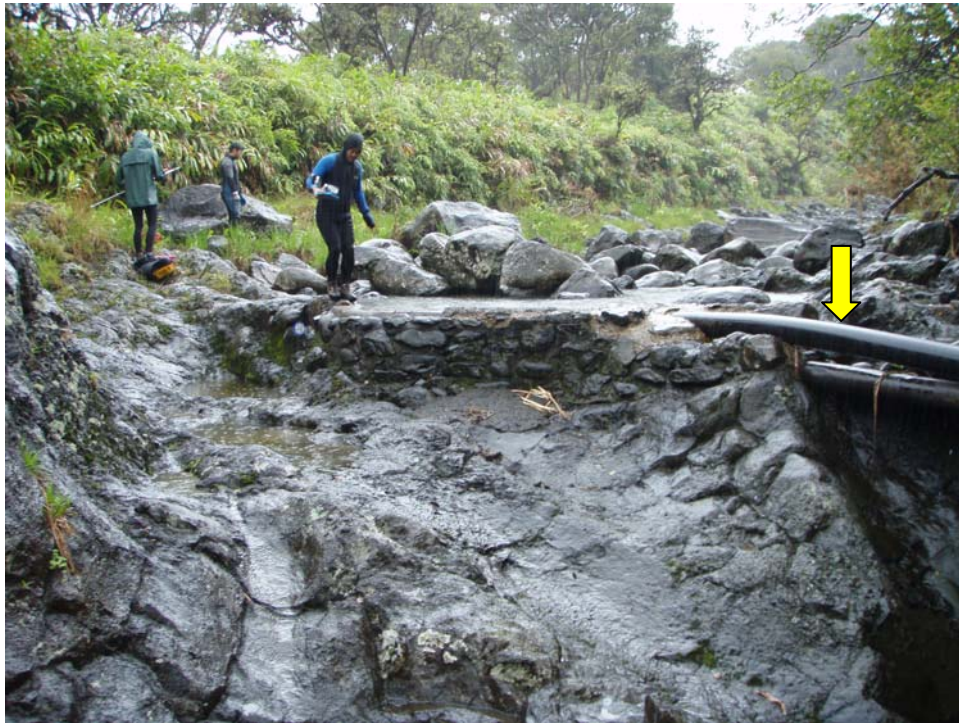
View upstream at next diversion from previous site gh063r-040208. Note 6" black PVC pipe (yellow arrow) on the right which is diverting water from the stream channel and carrying it downstream. Upper reach Pi'ina'au Stream, Maui, Hawai'i.
