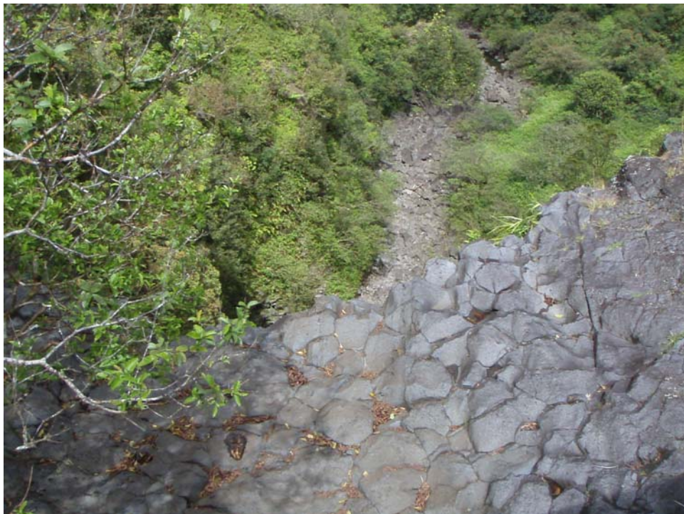
View downstream below the diversion bridge from site dk061n-040208. Note that the stream channel below is completely dry as the diversion structure spans the stream channel width. Upper reach Pi'ina'au Stream, Maui, Hawai'i.
