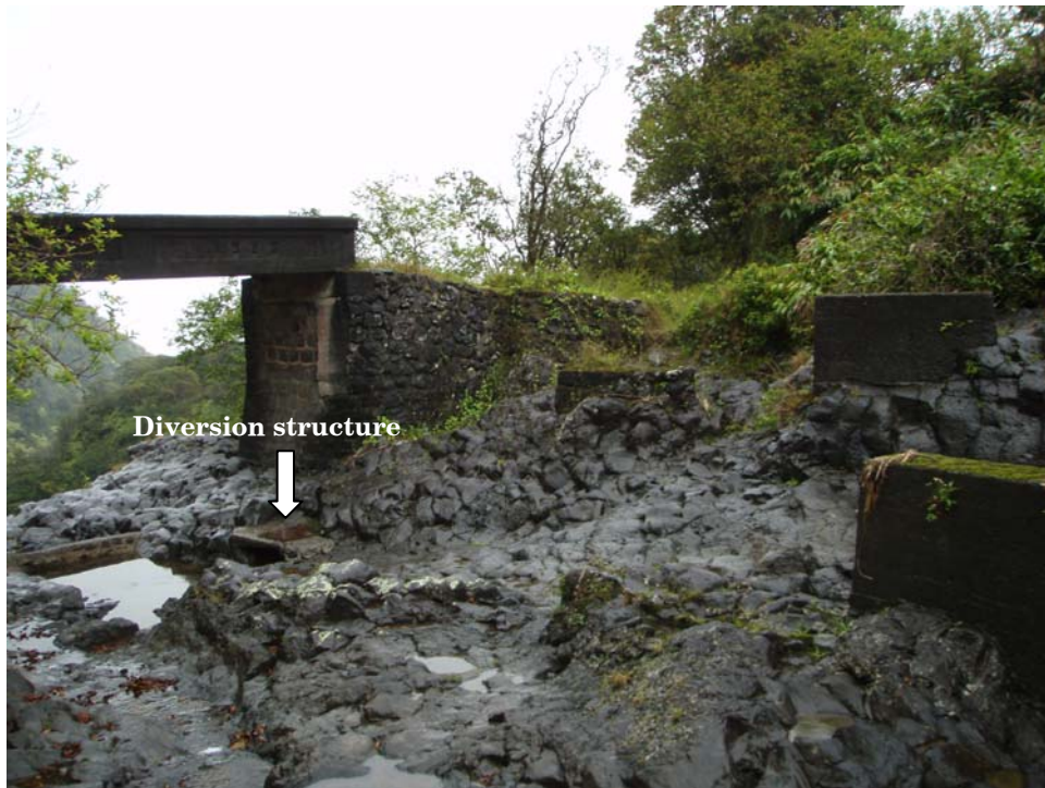
View downstream of diversion maintenance bridge and diversion structure below at site dk061n-040208. Upper reach Pi'ina'au Stream, Maui, Hawai'i.
